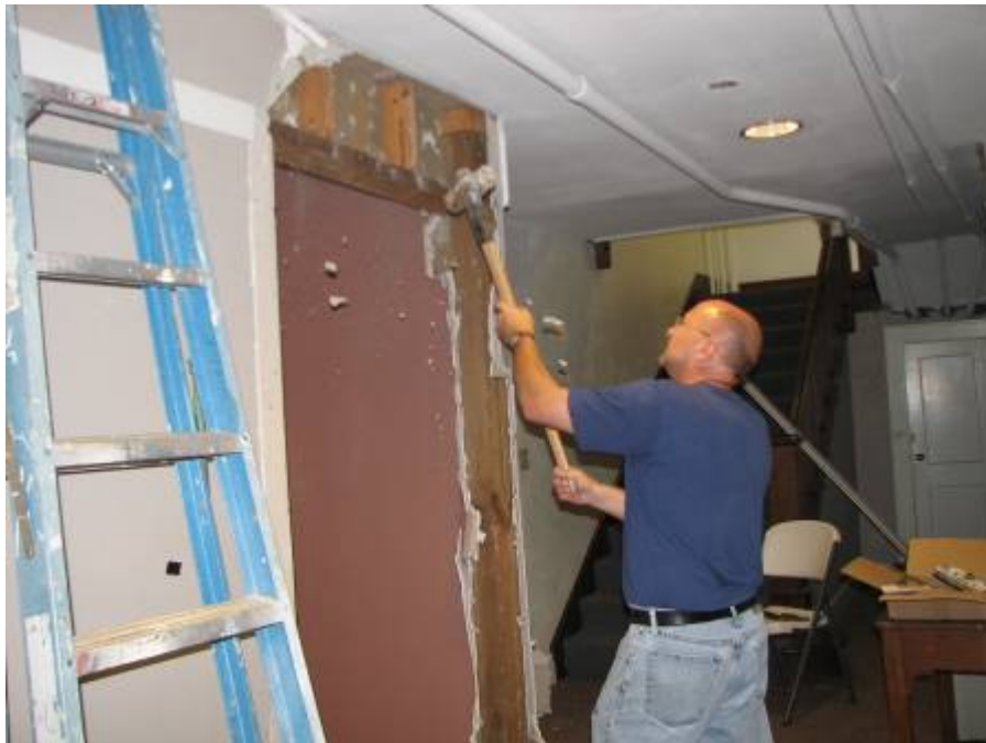
The walls in David's office come tumbling down to make way for the new foyer.
