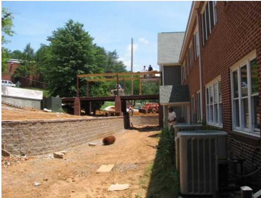
Members of our El Centro del Señor built the block wall and did a beautiful job.
