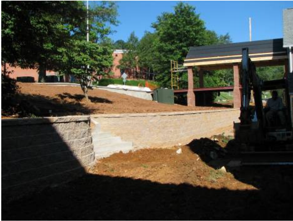
The roof is ready for shingles. The ground is leveled for sod.
