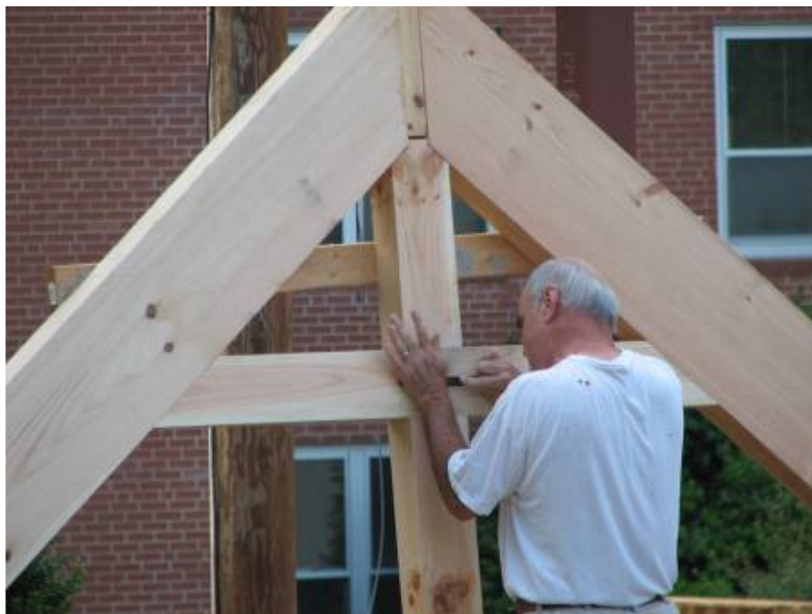
Robbie takes care of last minute details before the beams are raised in the air.
