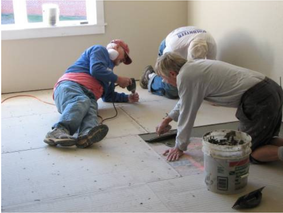
Bill, Robbie and Roy lay the backerboard in the new Wesley kitchen.
