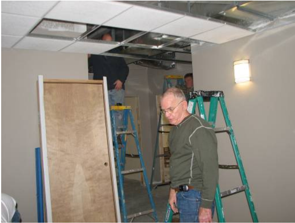
Ben came back from Florida for a week to install ceiling tile.
