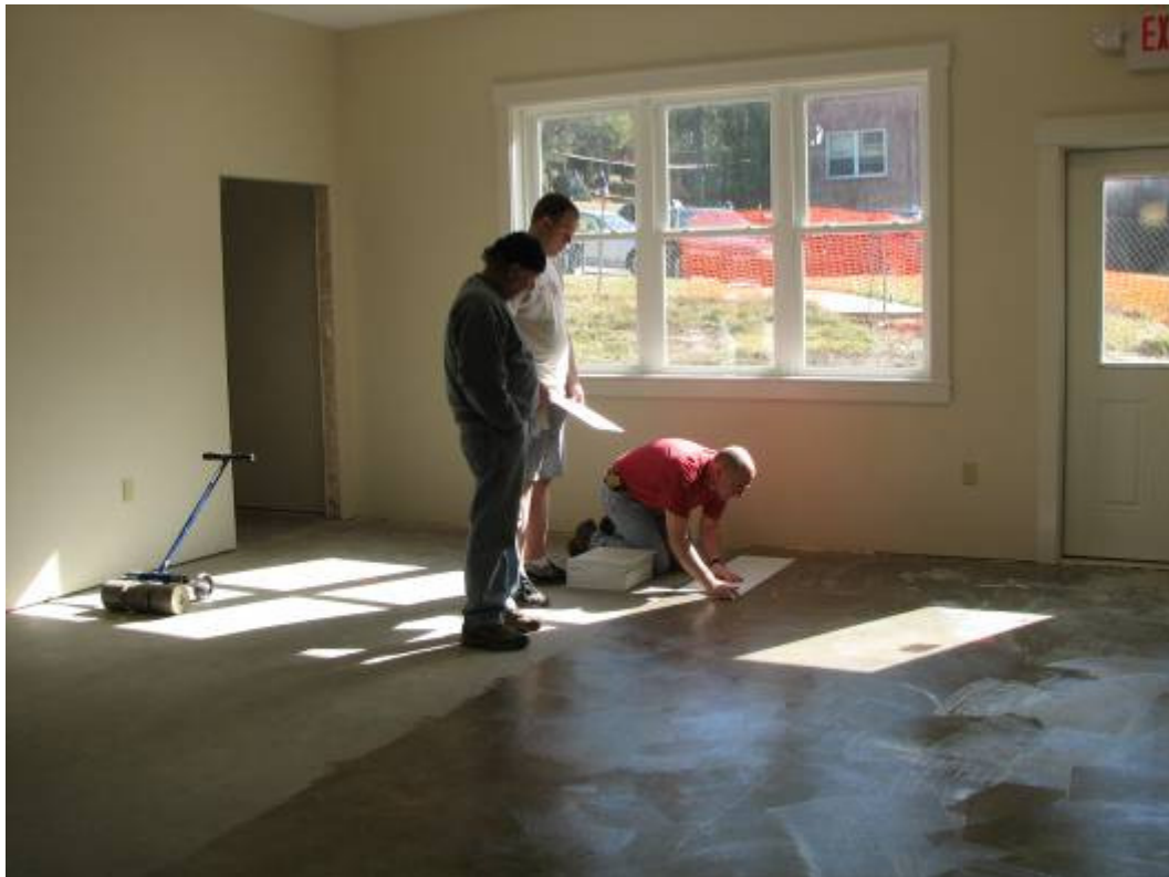
Dennis, Drew and David lay VCT (vinyl composition tile) in the new preschool rooms.
