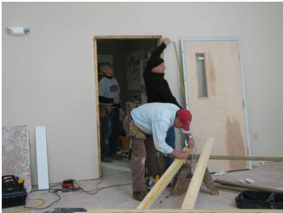
Roy, David and Lamar install a door in the new Wesley Center.
