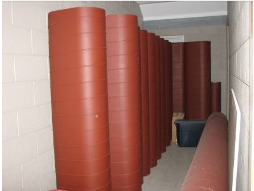
The HVAC duct work is all painted and ready to be installed.
