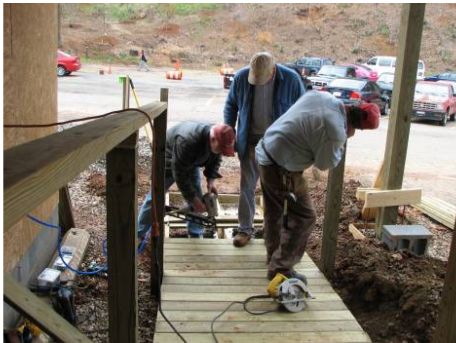
A temporary ramp is built for our new temporary entrance. Soon the old entrance will undergo excavation for an elevator, stairwell and Sunday school classroom.
