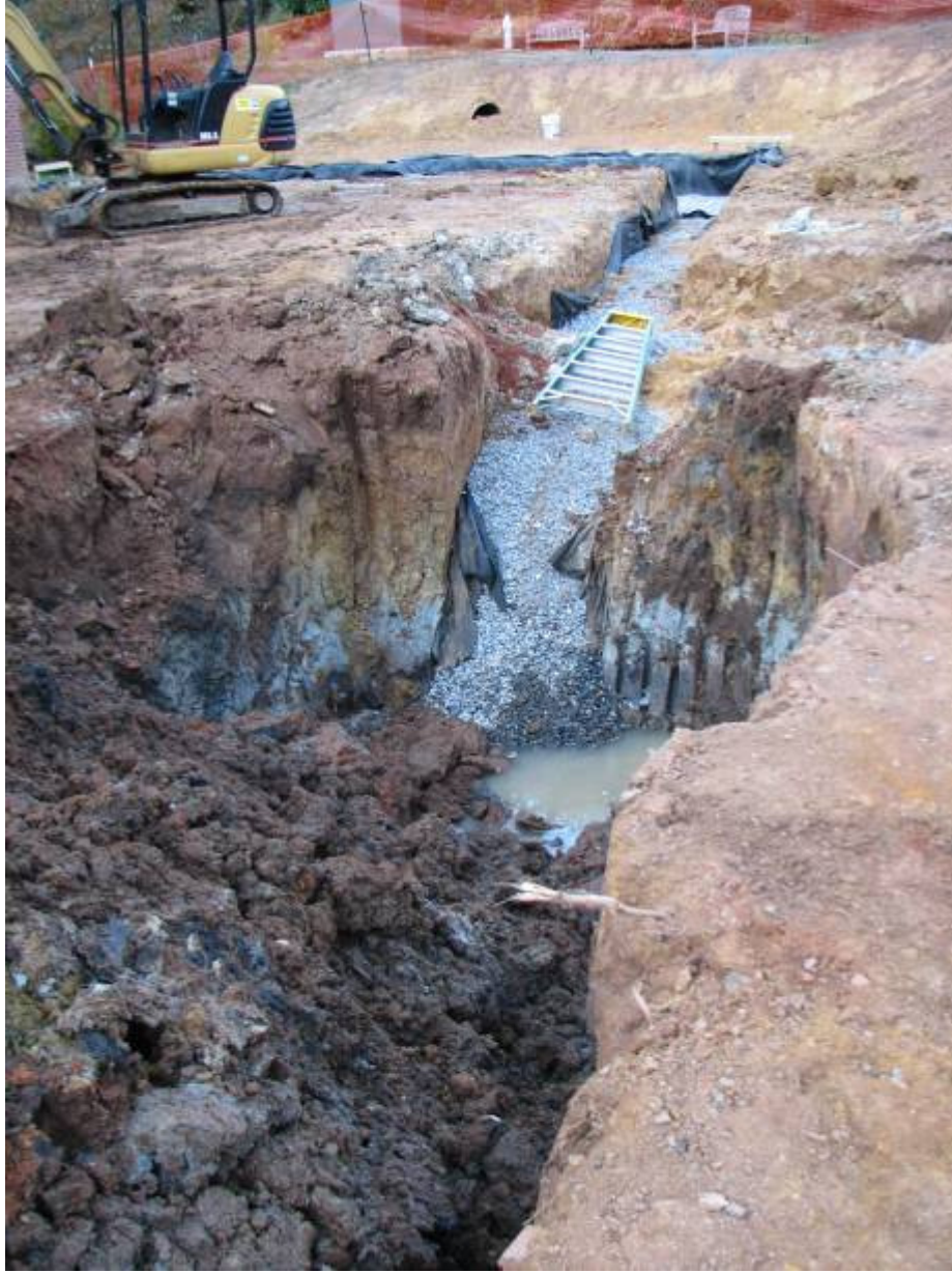
It certainly was neither a good day nor good news when this trench wall caved in.
